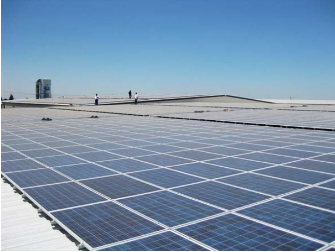
PV System at Minturn Nut Company
